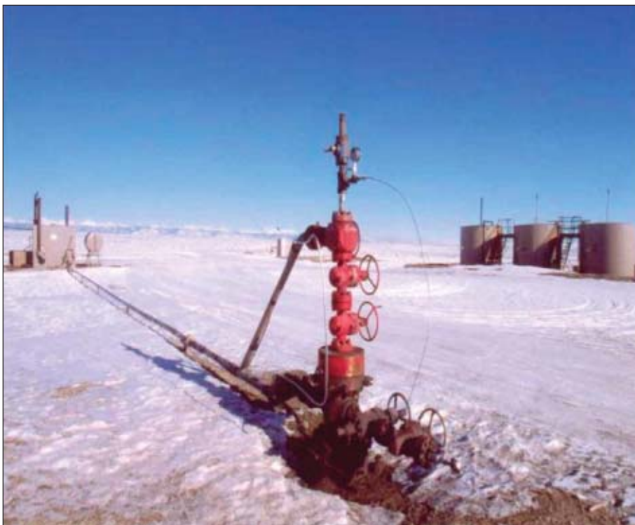
This single-well producing facility includes the wellhead in the foreground, with surface flowlines to an environmentally protected production building containing a heater and separator. In the far background is the electronic data gathering and transmission building. The three tanks, on the right, store condensate and water (Fig. 4). Photo from Shell.
