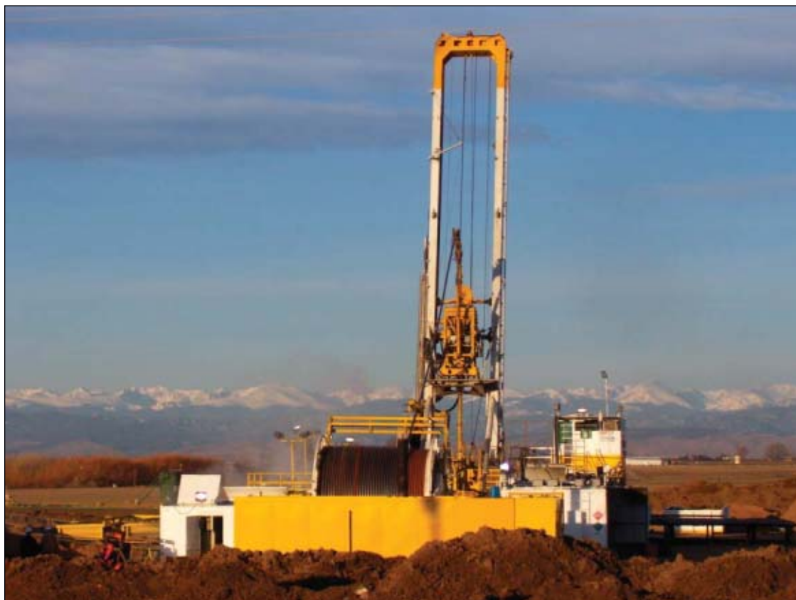
Xtreme's CT Rig 4, model 200DT, was drilling in the Denver-Julesburg basin near Greeley, Colo., in January 2007 for Anadarko Petroleum (Fig. 2; photo from Tenaris and Xtreme Coil Drilling).
